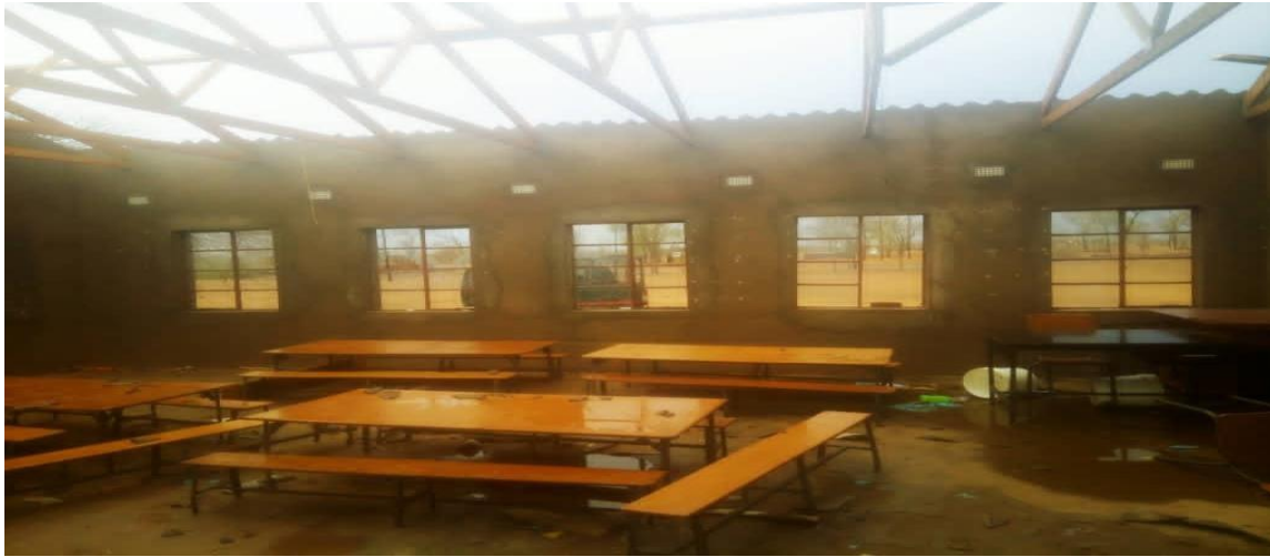
Plate 7.14-1: Pictures above show the effects of floods and hurricane like winds and storm in lower Muzarabani Kechu school Ward 7 Muvamba
